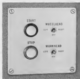
Figure 130A Electrical Panel at Right Side of Machine
